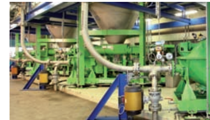
Solids pumps KOS 1050 in sewage works ProRheno (Basel, Switzerland)
