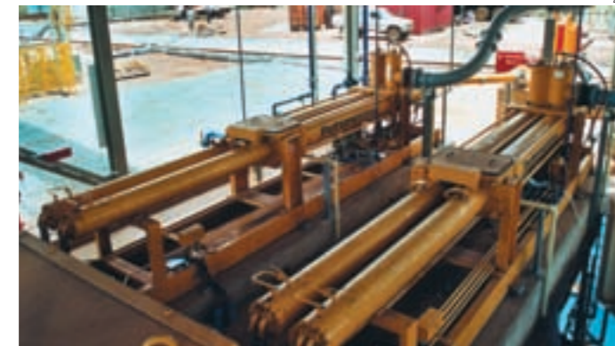
Two tailings pumps HSP 25100 at the Bulyanhulu goldmine (Tanzania)
