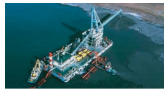
Three huge piston pumps KOS 25100 und 25200 are pumping silt out of the sea for arising an artificial island in front of the Japanese coast line
