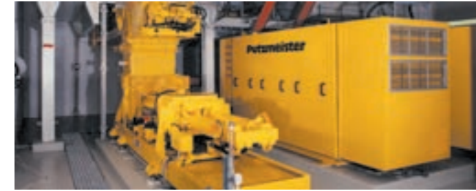
Co-incineration of sewage sludge in the coal-fuelled power station Zolling (Germany): solids pump KOS 2180
