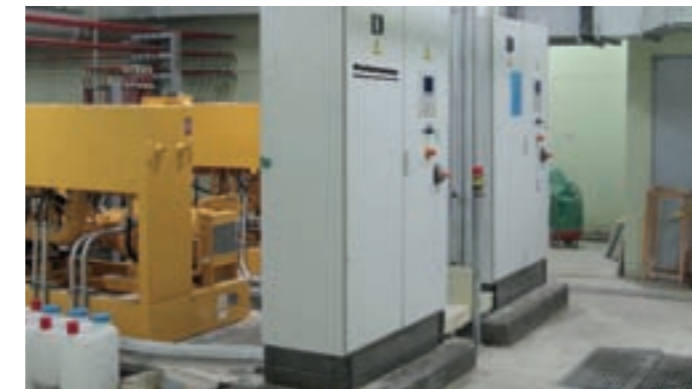
Local control panel at the wastewater treatment plant Gulpocheon South Korea
