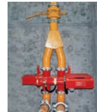
ZX 150 IP line in an incinerator plant
