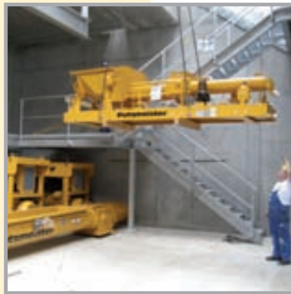
New installation in the sewage treatment plant, Neu-Ulm, Germany
